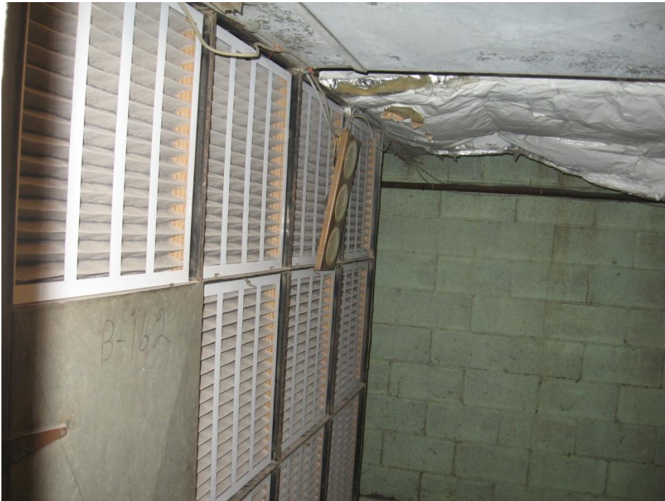
Photo 4: Fiberglass Insulation in Return Air Compartment
