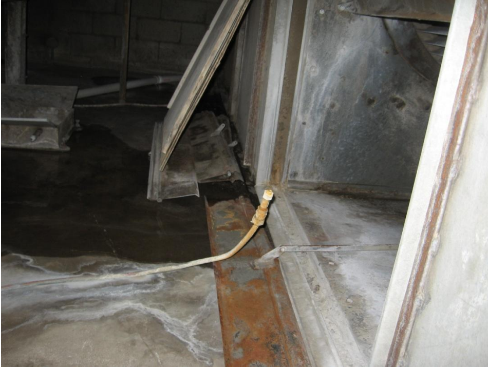
Photo 3: Spray Nozzle used to Humidify Air – Note Water on Plenum Floor in Background
