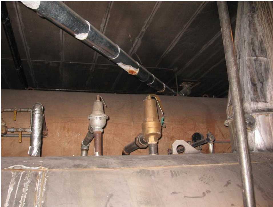
Photo 1: Long Horizontal Hot Water Heater Exhaust Flue Pipe
