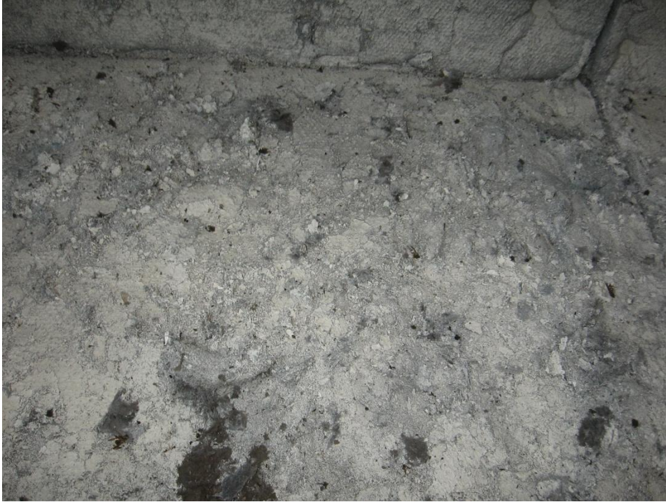
Photo 6: Worn Fiberglass Insulation inside Mixed Air Compartment of AHU
