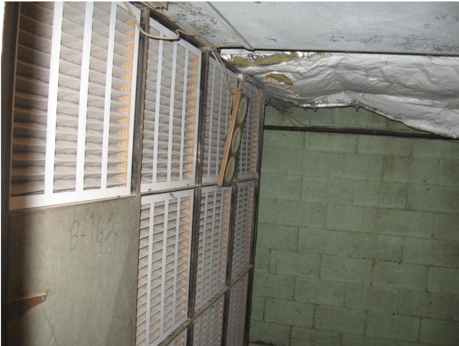
Photo 4: Fiberglass Insulation in Return Air Compartment
