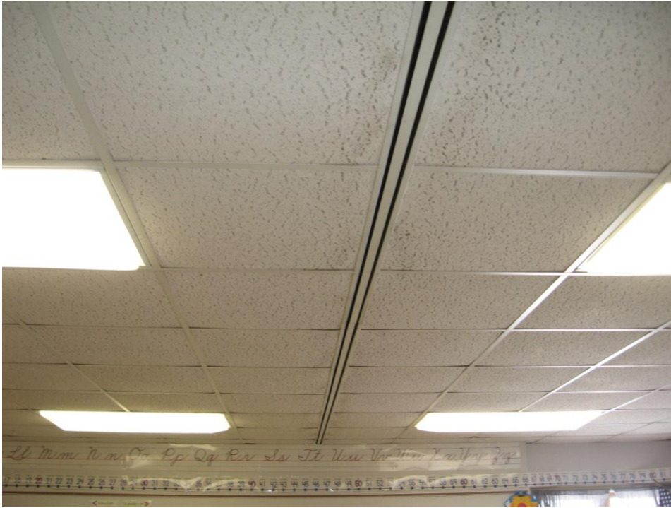
Photo 5: Single Linear Air Supply Diffuser in Elementary Classrooms
