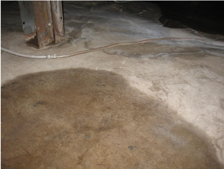
Photo 2: Areas of Moisture and Moisture Staining on Floor of Plenum
