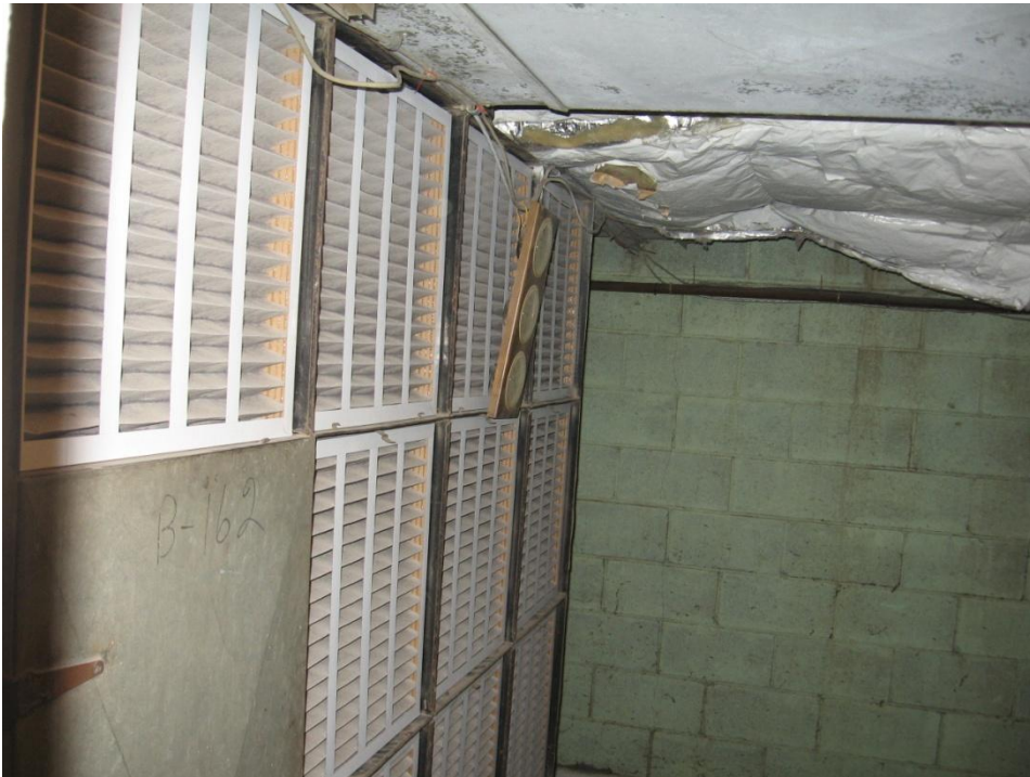
Photo 4: Fiberglass Insulation in Return Air Compartment
