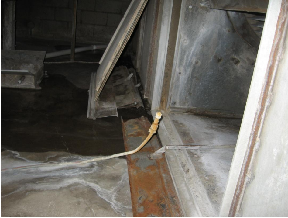
Photo 3: Spray Nozzle used to Humidify Air – Note Water on Plenum Floor in Background
